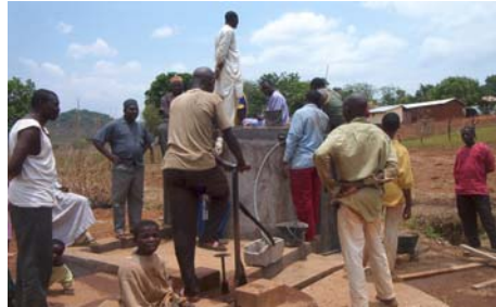
Water is pumped directly from the well to the slow sand filter unit
