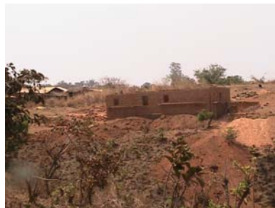
Mud blocks have been laid for the construction of a Fulbe youth hostel
