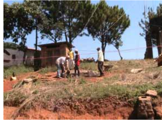
Chad helps mix concrete by hand as the anchors are prepared for the antenna tower cables
